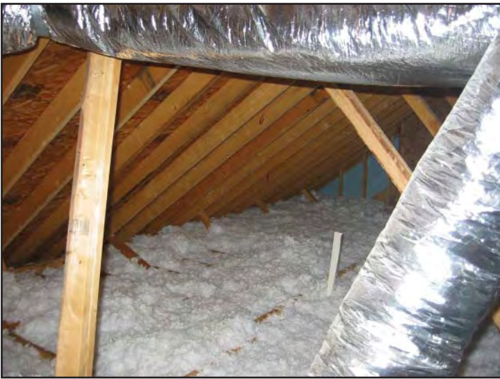
Figure 7.2. Blown Attic Insulation
