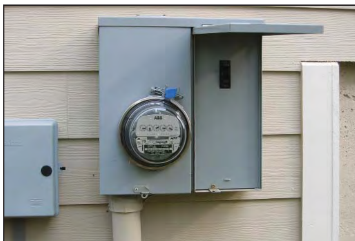
Figure 11.15. External Power Shutoff and Meter
