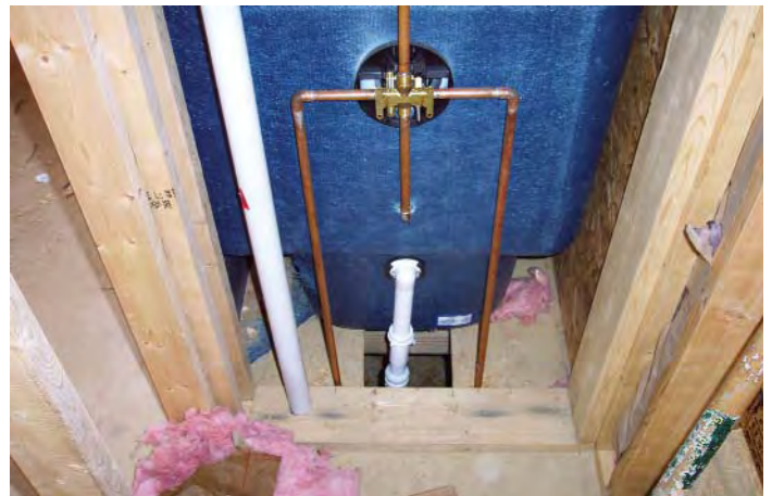
D. Mixing and antiscald water flow control, vent for fixture, hot and cold water lines, and bathtub overflow shown. At this point in construction, insulation might be considered for the hot water lines. Water service and waste water line.
