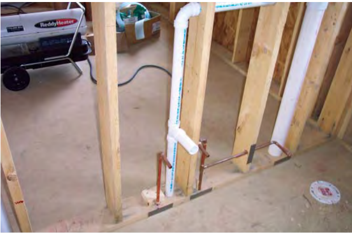
C. Vent for the sink and toilet, soil pipe, and cap for toilet connection shown. A wax or plastic seal shaped like a donut will be placed on the cap before bolting down the toilet.
