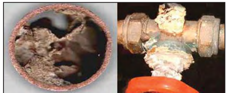
Figure 7.6. Corrosion in Piping Resulting From Galvanic Response
