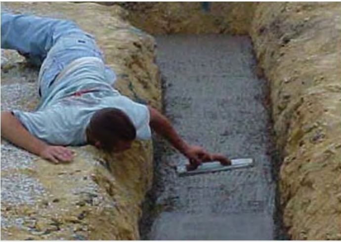
B. The concrete on top of the footer is leveled to establish a surface for the foundation of the home. Once the footer has hardened, the perforated drainage pipe will be laid on the outside of the poured foundation wall. The reinforcing rods were positioned in the trench before pouring the concrete.
