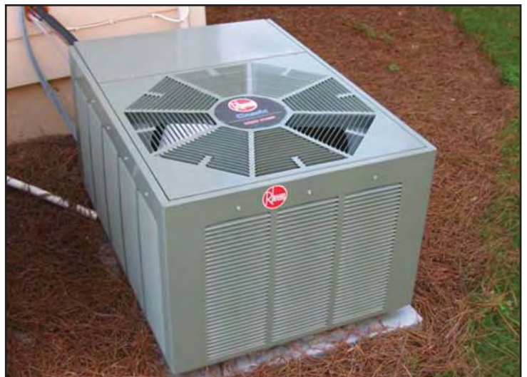
Figure 12.21. External Air-conditioning Condenser Unit
