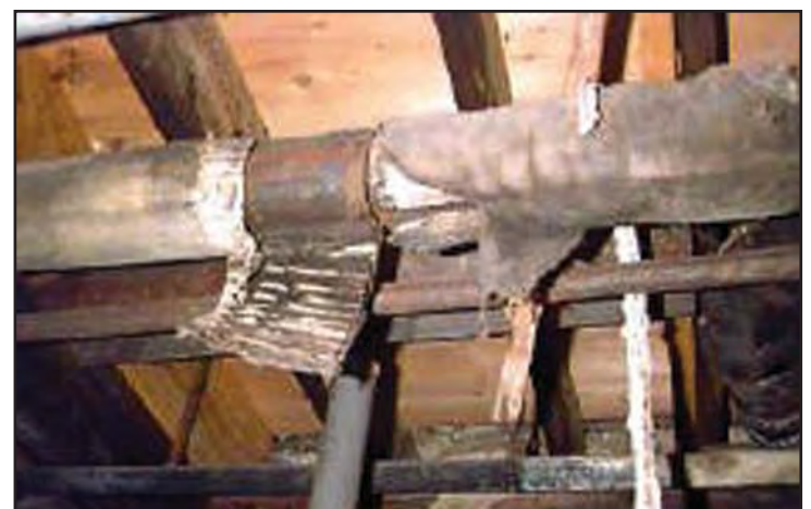
Figure 12.6. Heating Ducts Covered With Asbestos Insulation
