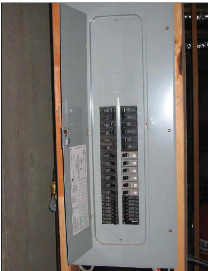
Figure 11.14. 200-Amp Service Box
