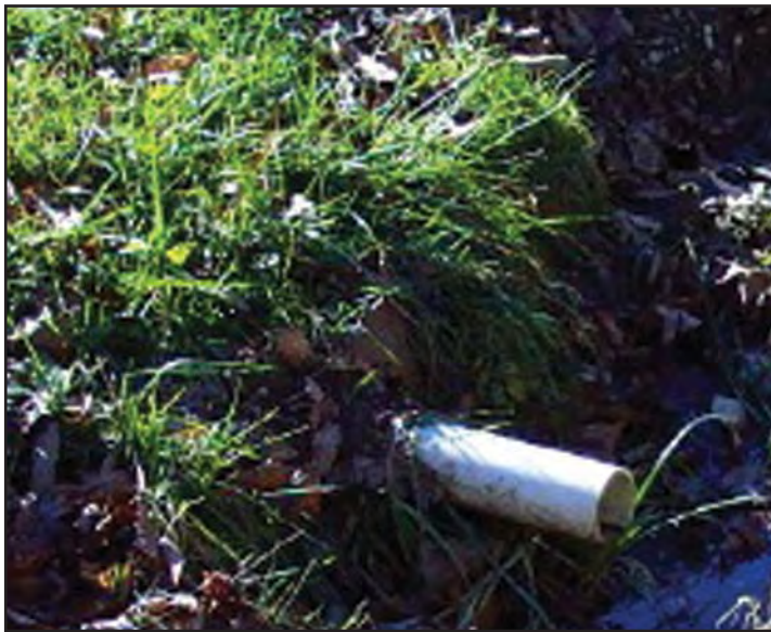
Figure 10.2. Straight Pipe Discharge Source: Donald Johnson; used with permission.
