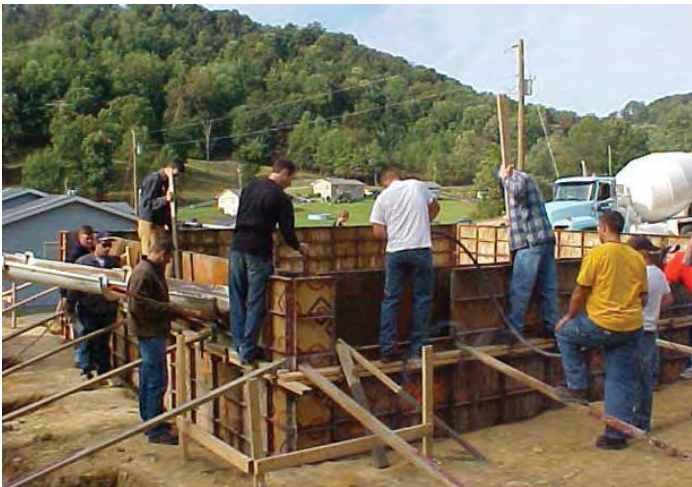
D. Foundations are not always poured concrete, but are often cinderblock or similar materials that are cemented in place to form the load-bearing wall. The arrow shows the concrete chute delivering concrete into the form. Long poles are pushed into the freshly poured concrete to remove air pockets that would weaken the foundation.
